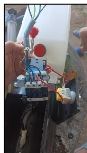
Fig. 1.9: wrongly connected DOL motor starter
